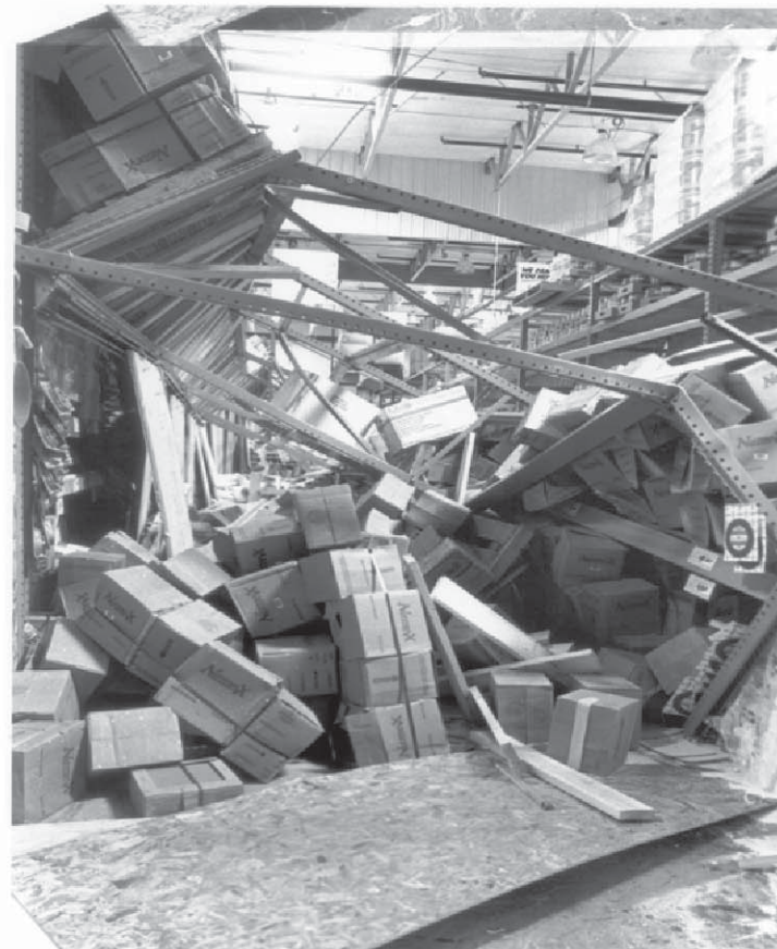
Figure 2-2 Cross-aisle collapse in the tile section of the Santa Clarita store.
