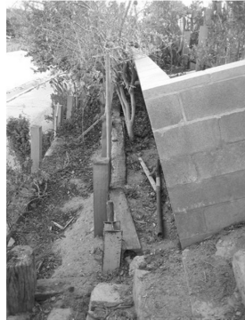
Failure of an unpermitted retaining wall.
