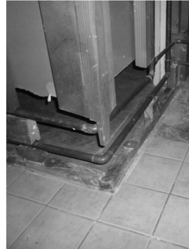
Framing cut during an unpermitted re-pipe.
