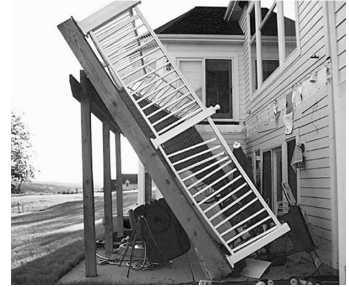
Deck collapse due to inadequate connections.
