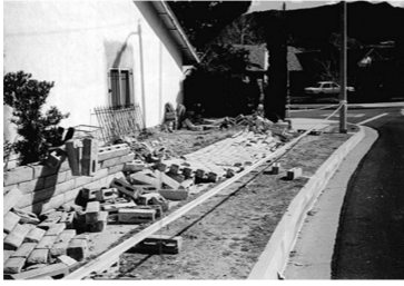
Unpermitted block wall which collapsed in the 1994 Northridge Earthquake.
