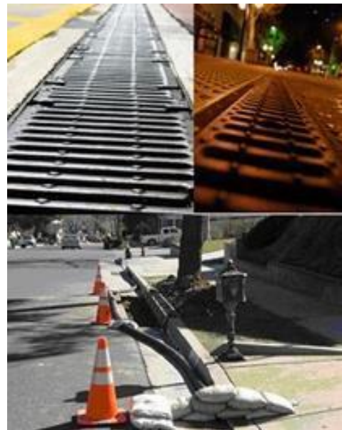
Figure 11: Storm Drain Debris Mitigation
