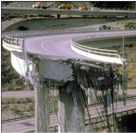
Figure 4: Freeway Collapsed Interchange
