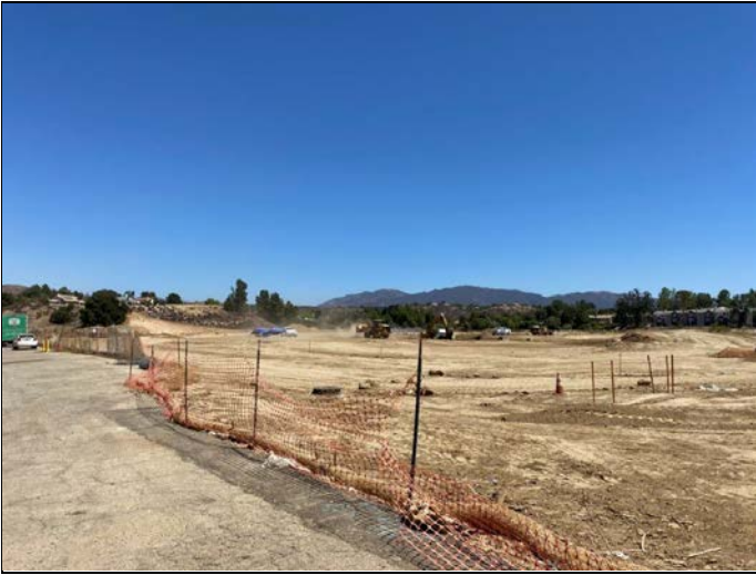
1. View of the subject property and active storm drainage and grading work
