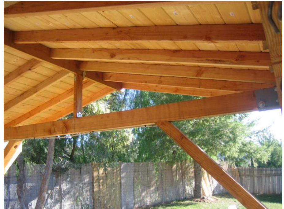
(No lateral load path. Undersized beam.)
