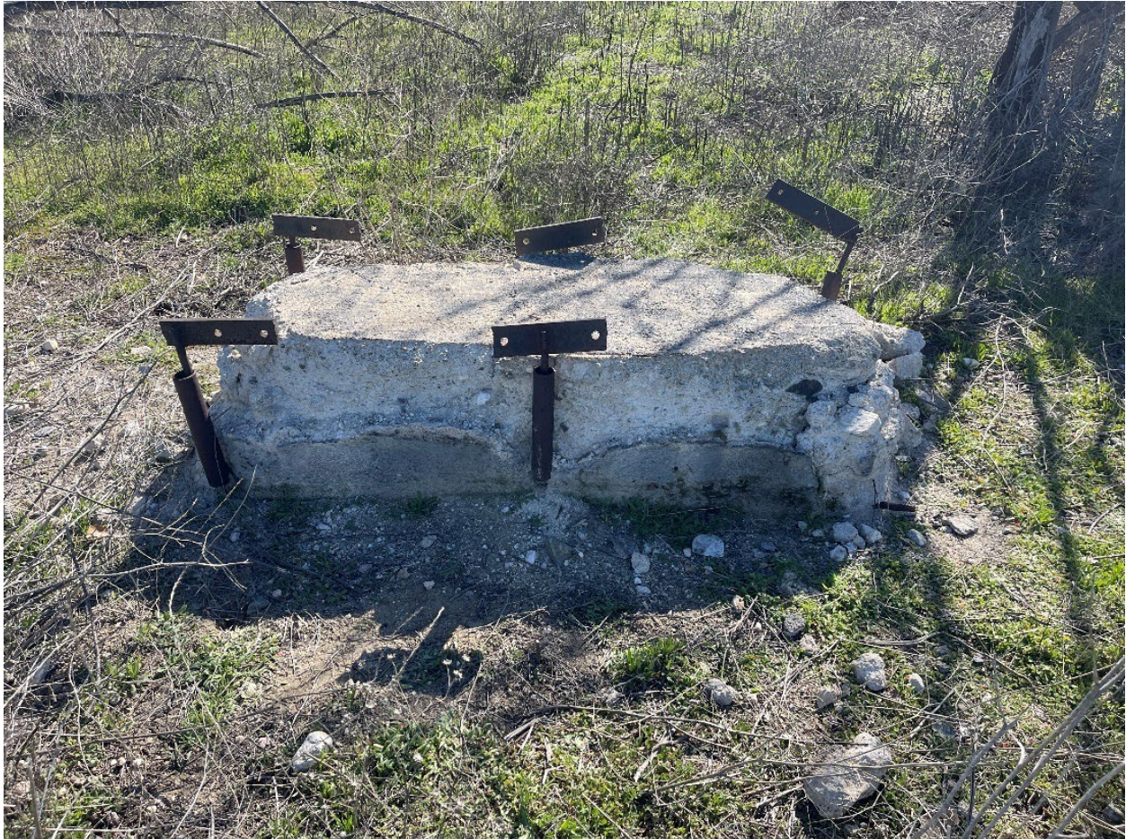
Photo 5. MBI-VP-MY-01H Feature 5 - Concrete remnant with metal brackets.
