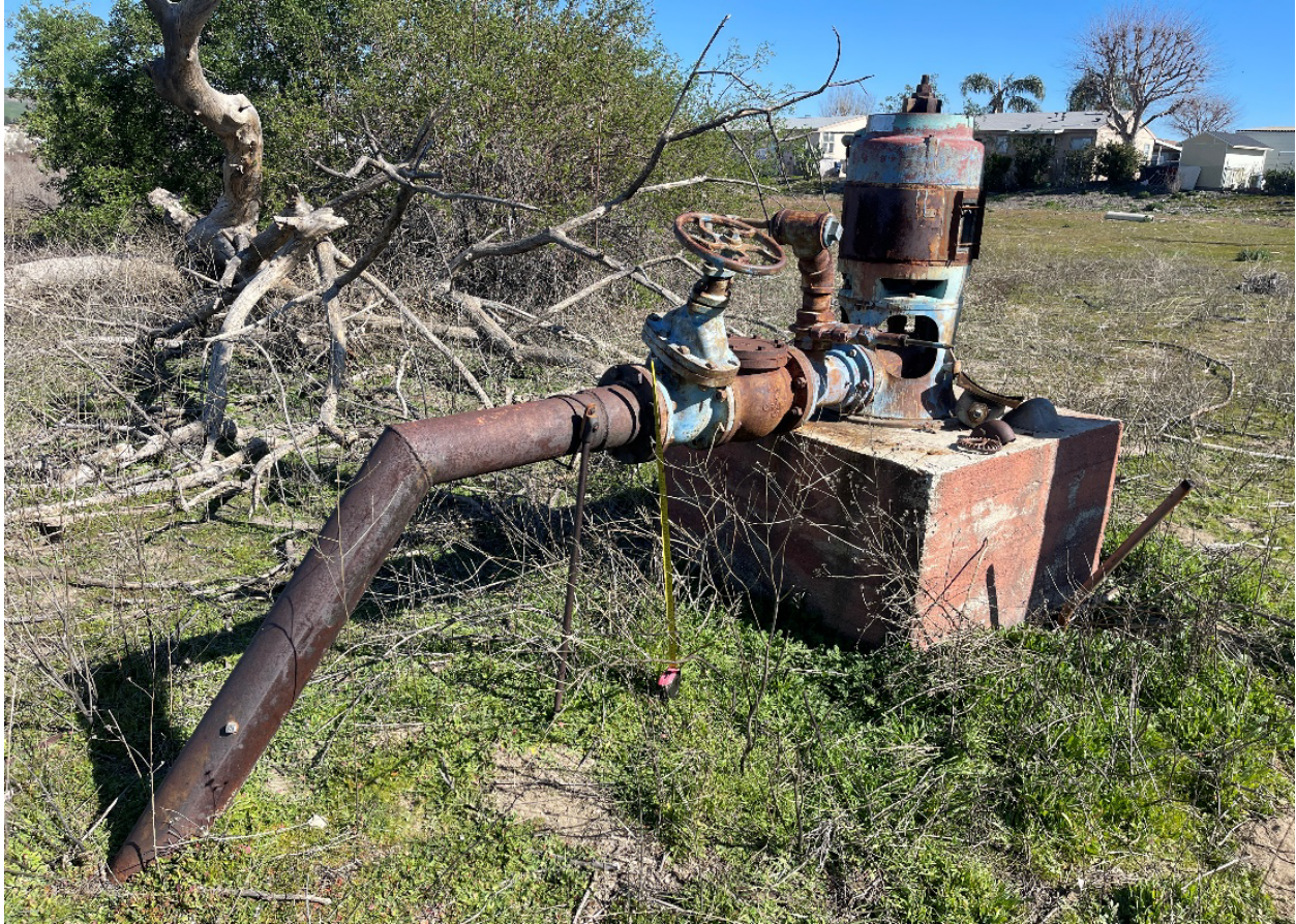
Photo 3. MBI-VP-MY-01H Feature 3 - Turbine water well pump on a concrete block with associated valves and pipes.
